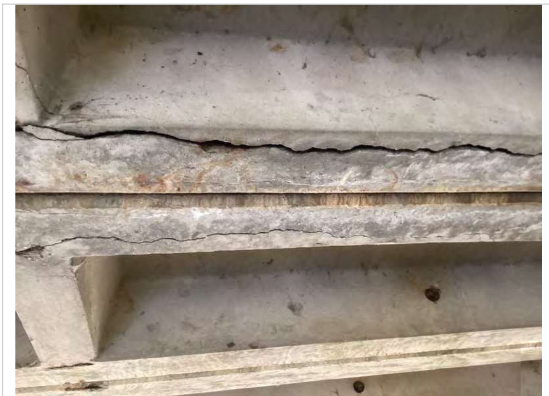
Span 2 slab D impending spall
