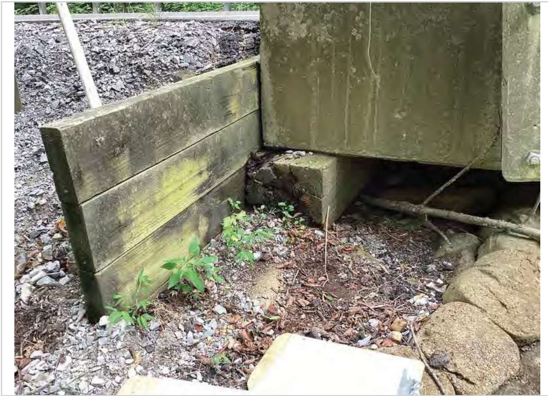
Abutment #1 right end cap decay
