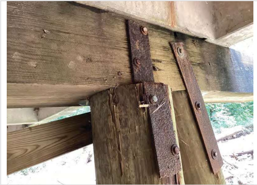
Bent #2 splice plates corrosion (typical for bents #1 and #2)
