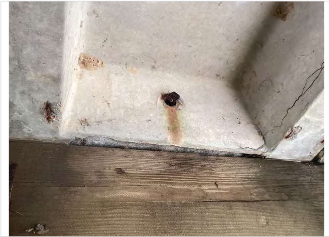
Span 2 span connectors corroded. 7 nuts missing
