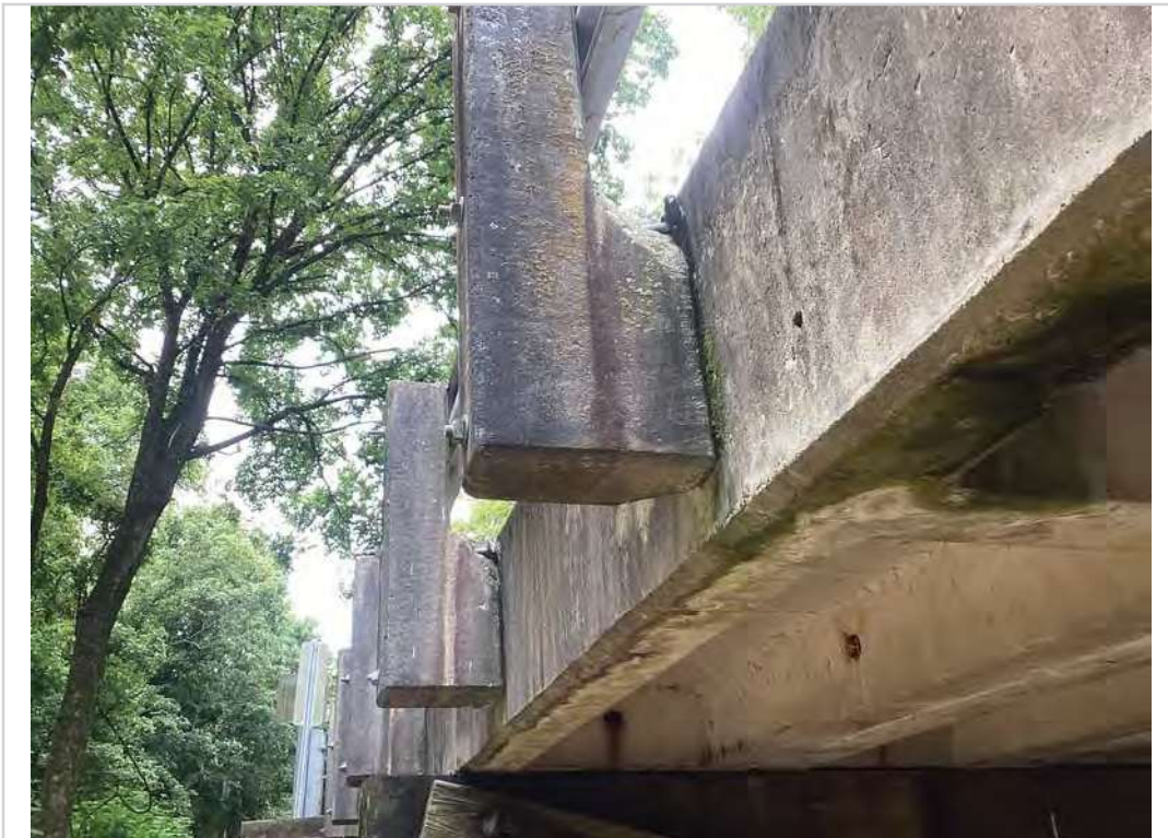
Span 2 right side posts damaged
