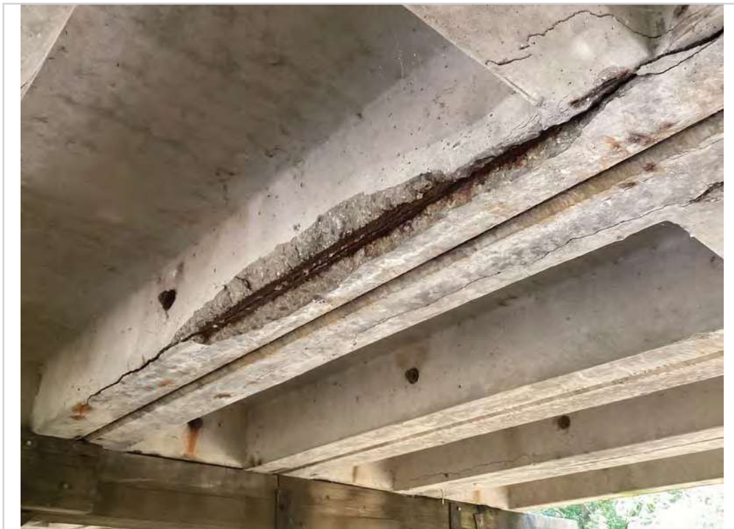
Span 2 slab D spall to steel
