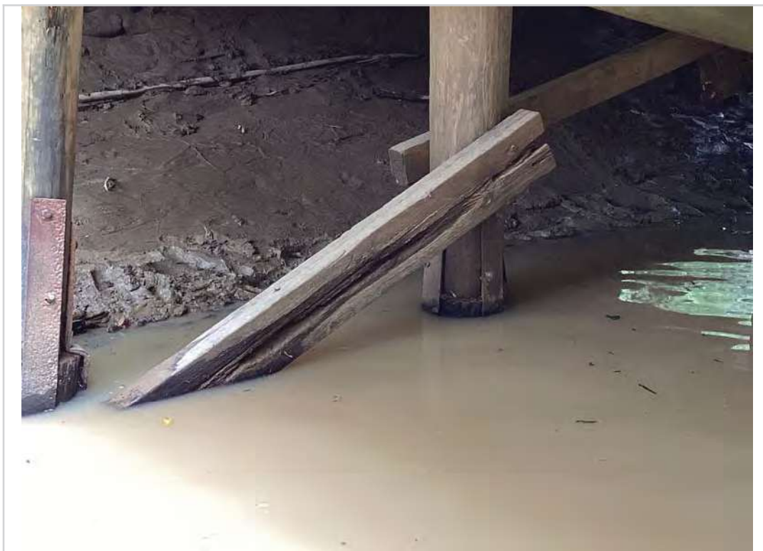
Bent #1 bracing decay (typical for bents 1 and 2)
