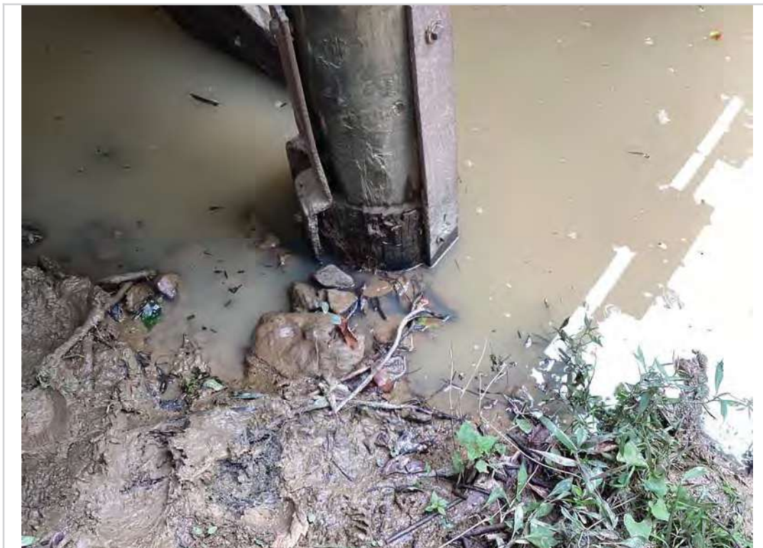
Bent #1 pile E decay
