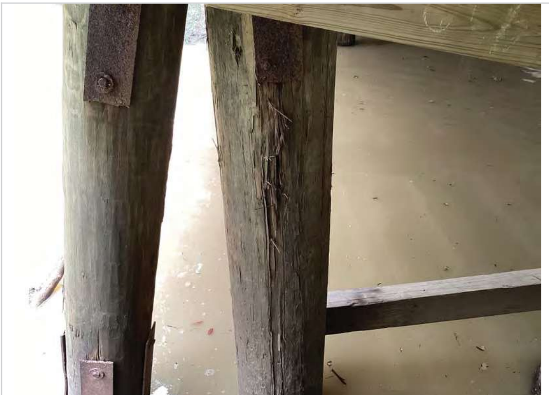
Bent #2 pile E splintering
