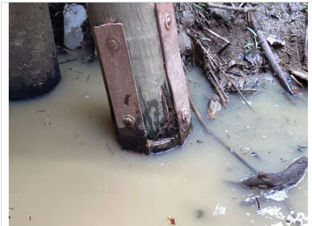
Bent #2 pile E decay
