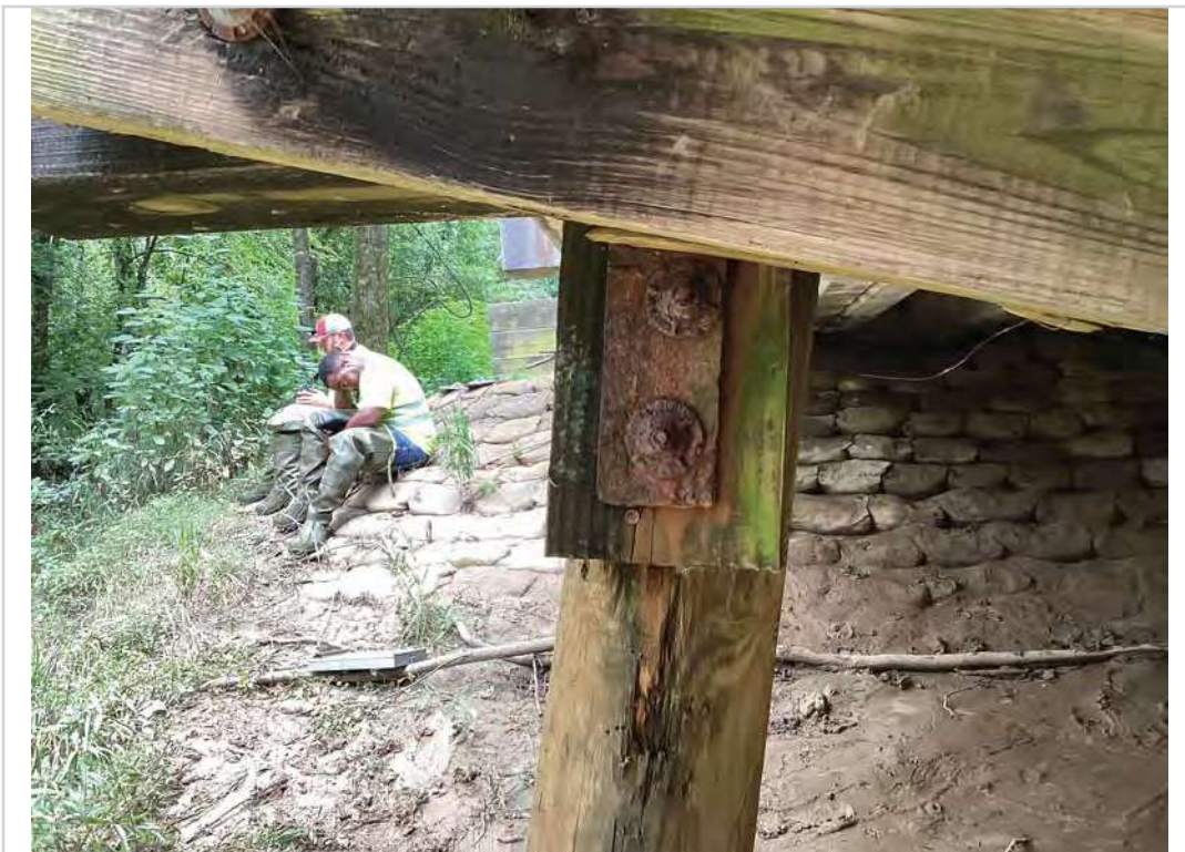
Bent #1 splice plates corroded
