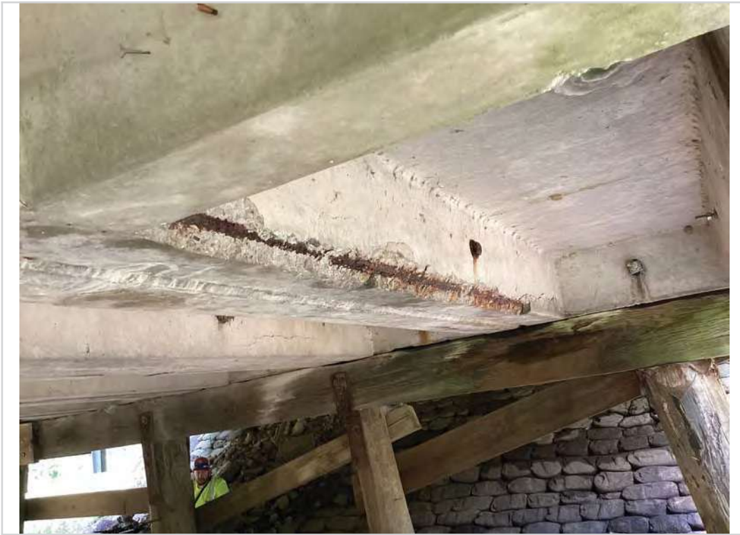
Span #3 PCCS "G" spall to steel
