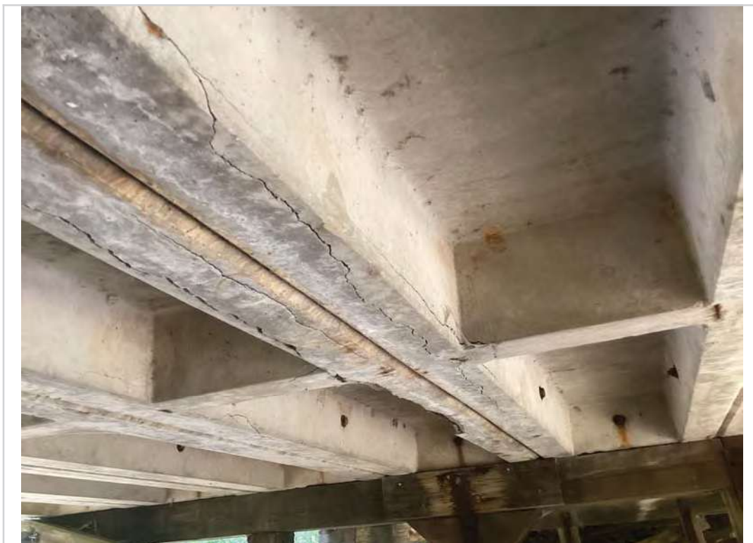
Span 2 slab E impending spall
